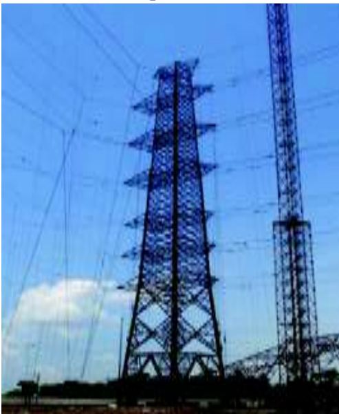
220kV Transmission Tower
