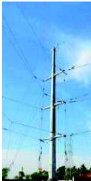
400kV D/C Quad Moose Monopole
