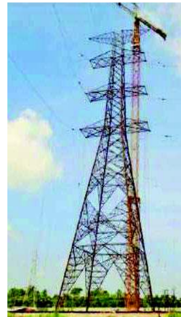
500kV Transmission Tower
