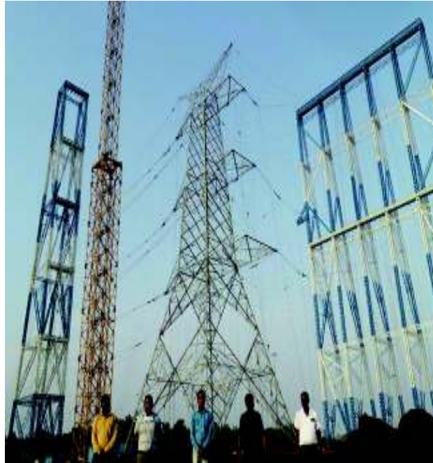
765kV Transmission Tower
