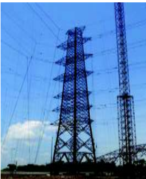
220kV Transmission Tower
