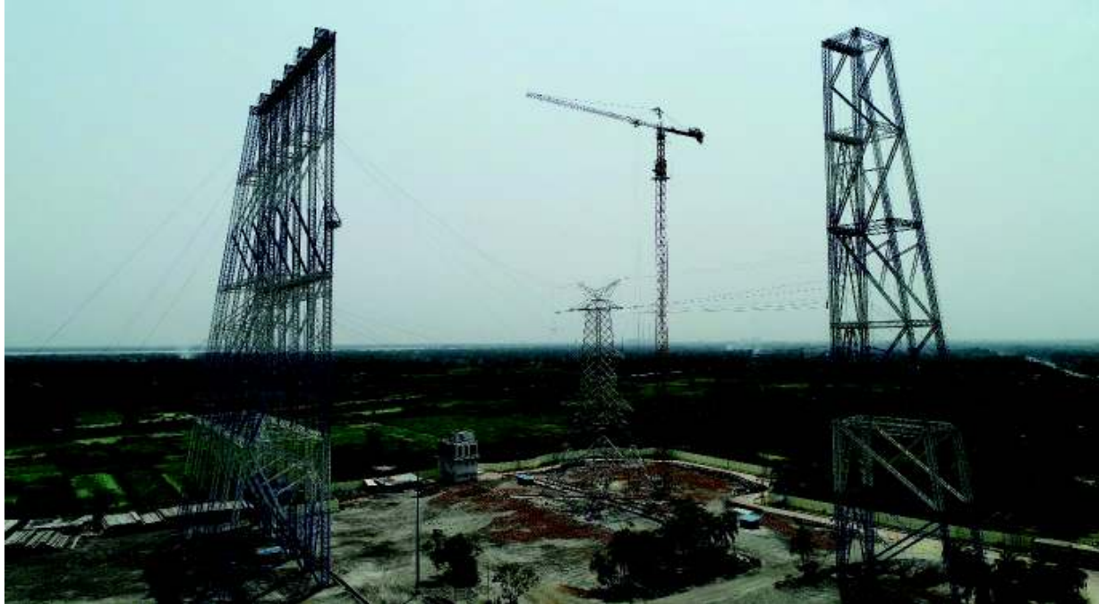
Transmission Line Testing Station
