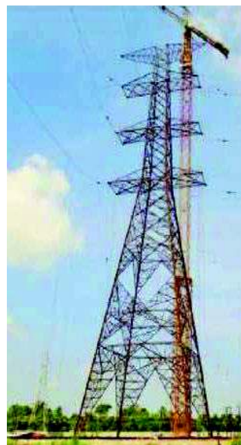
500kV Transmission Tower
