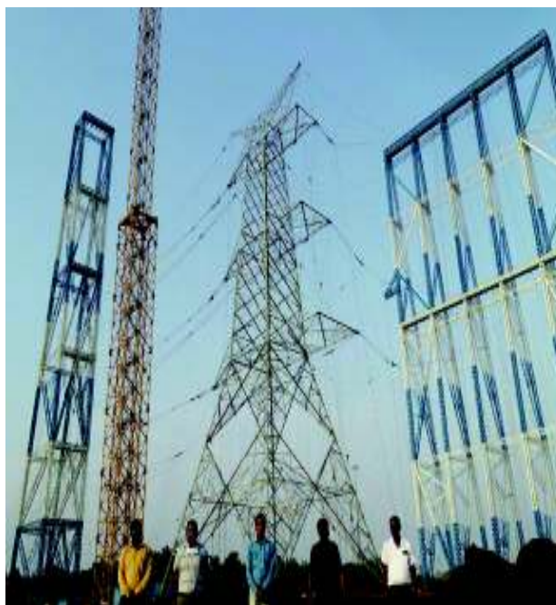
765kV Transmission Tower
