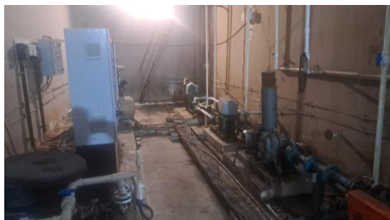
Internal View of STP in Subject Project
