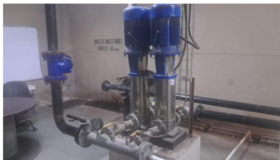
Internal View of Water Pump Room in Subject Project
