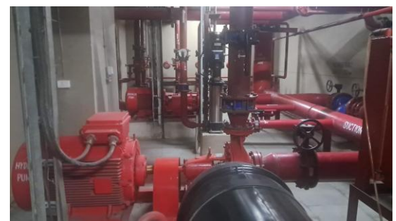
Internal View of Fire Pump Room in Subject Project
