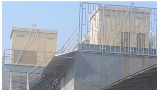
View of transformers at Subject Project
