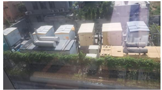
View of DG Sets Yard at Subject Project
